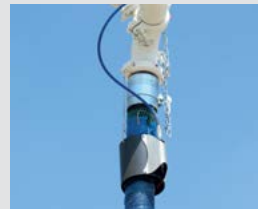
Shut Off valve in pipeline
